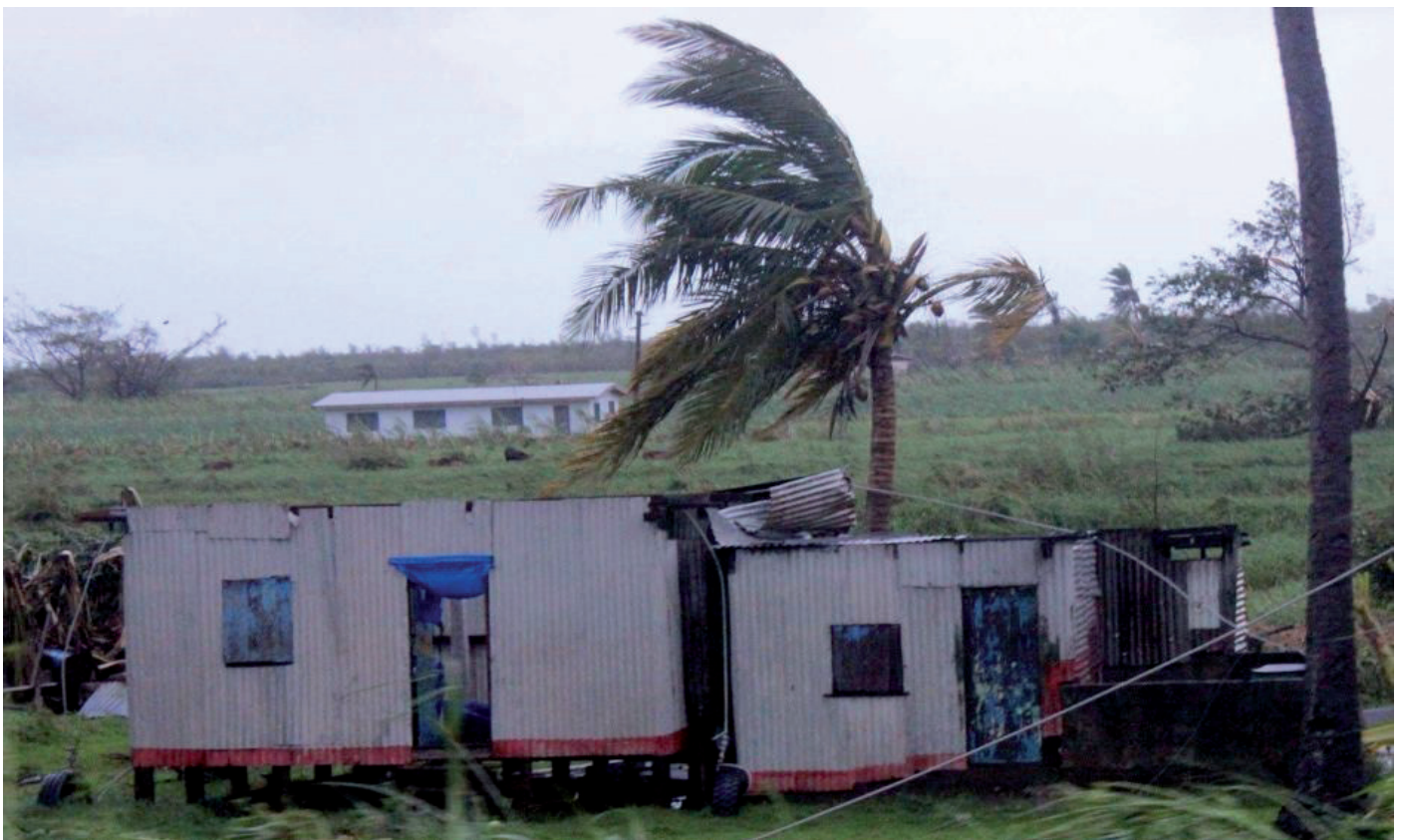
Damage after Tropical Cyclone Winston, Feb 2016, source: www.abc.net.au
