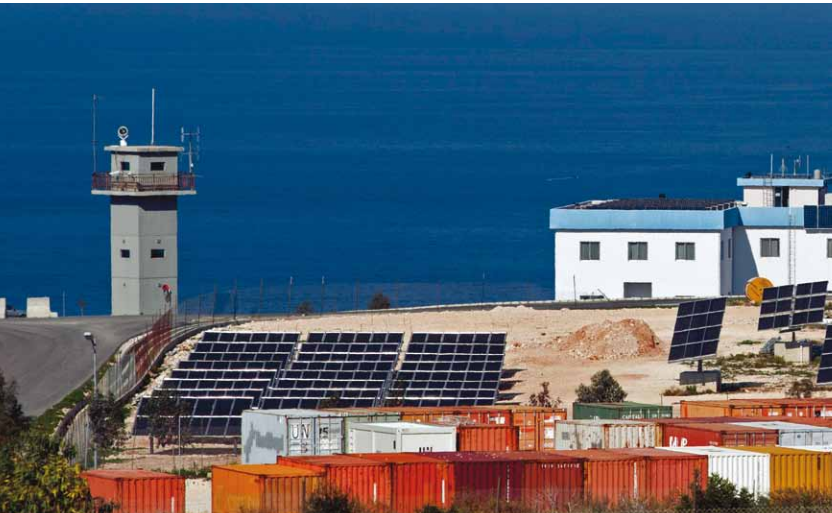
Fig. 3. A view of solar panels on the UN Interim Force Base in Lebanon (UNIFIL). Naqoura, Lebanon. © UN Photo/Pasqual Gorriz.
